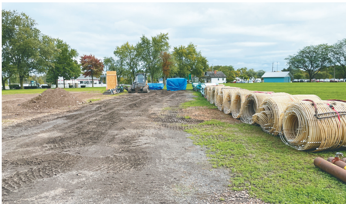
Residents and passersby have noticed work underway in the Village of Lewiston. At top, the St. Peter R.C. Church rectory is getting an exterior makeover. Above, materials have started arriving for the Lewiston Family Ice Rink at Academy Park.
